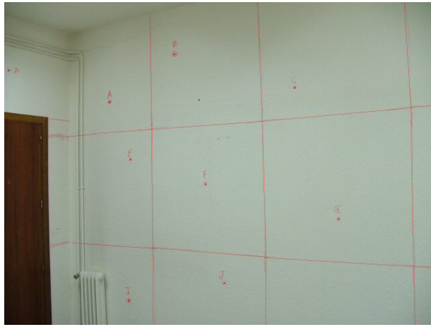
Figure 2 – Partial view of receiving room
