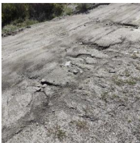
Figure 21. Transverse erosion on the unpaved EBVT at Montesinho in 2023 (Kolodi 2023)
