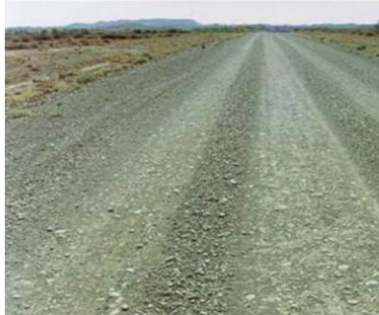
Figure 18. Photograph of an unpaved road with loose aggregate on its surface (Australian Road Research Board. 2009)
