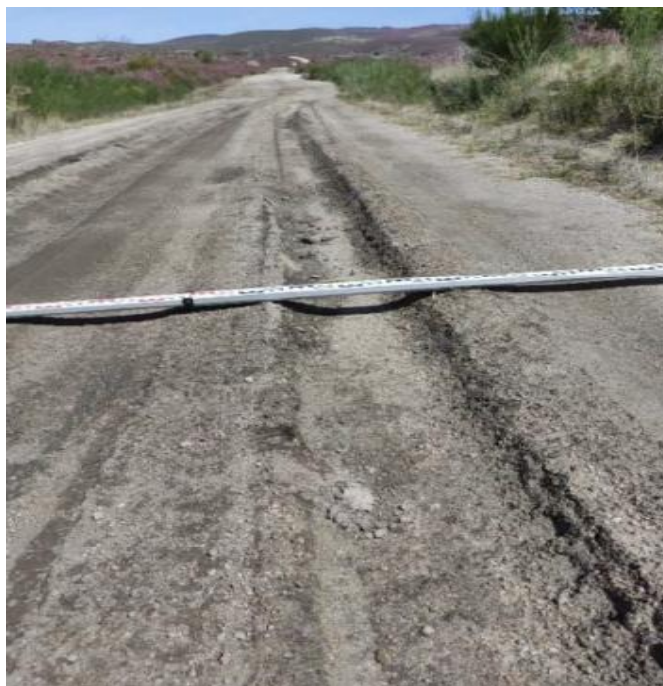
Figure 15. Example of subsidence on the unpaved EBVT at Montesinho (Kolodi 2023)
