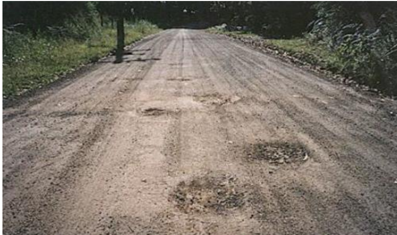
Figure 17. Photograph of an unpaved road with potholes on its surface (Australian Road Research Board. 2009)
