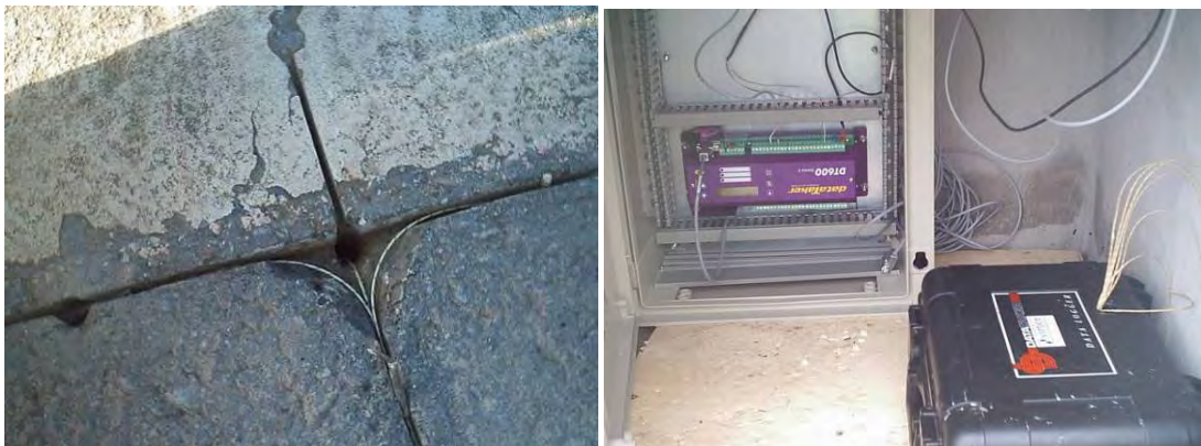
Figure 2. Pavement instrumentation and data acquisition
