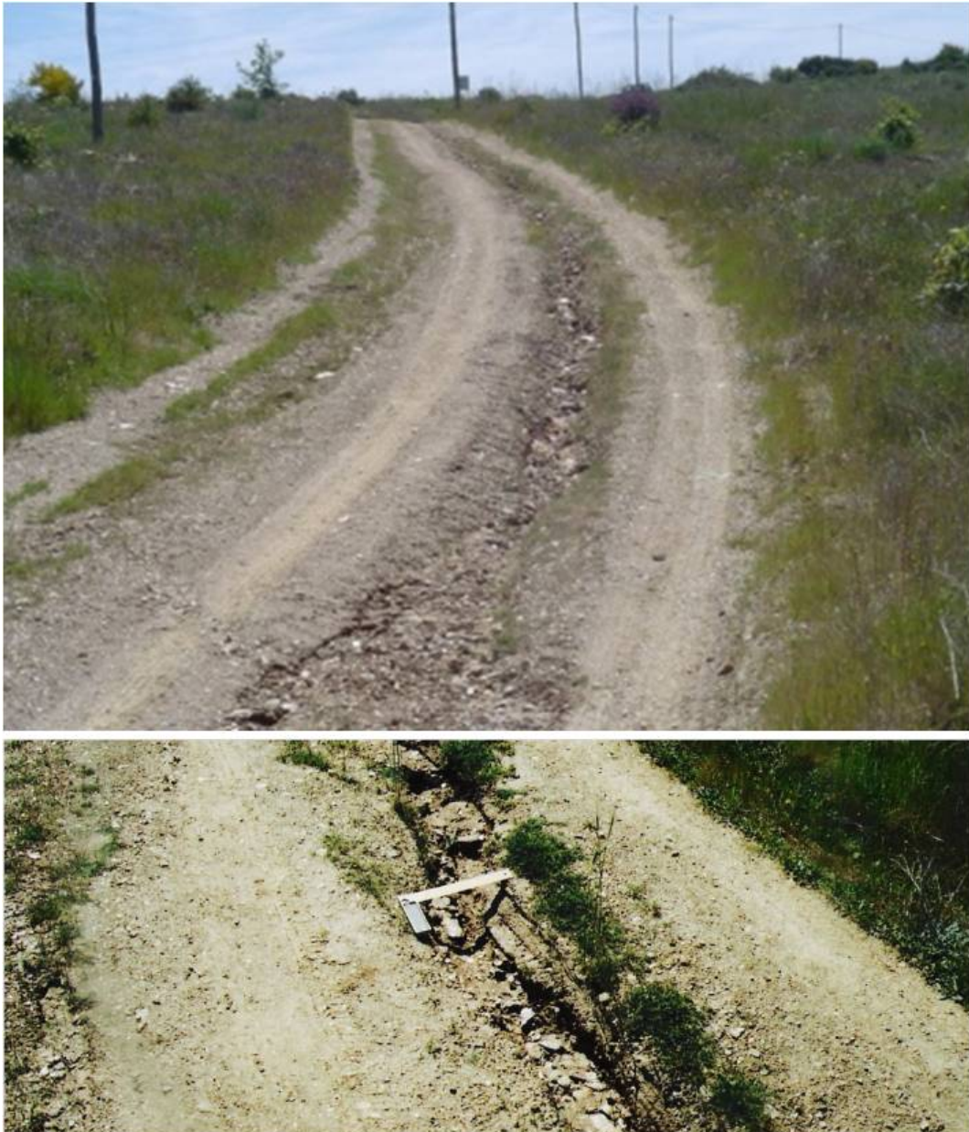
Fig. 3.7: Measuring a rilled forest road (Lamas de Podence).
