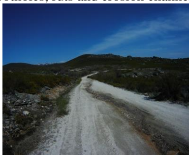
(a) Erosion channel.
