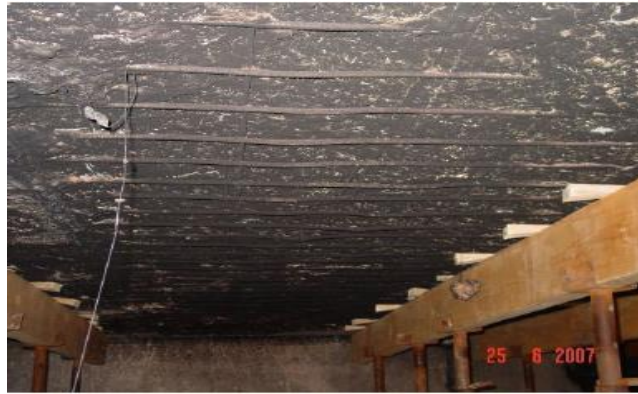
Figure 9 - The Apartment building Geleen after fire [24].
