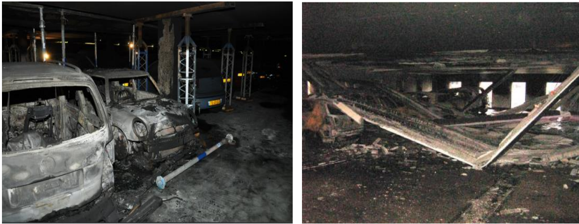
Figure 11 - The open car parking of building Harbour Edge after fire [26].
