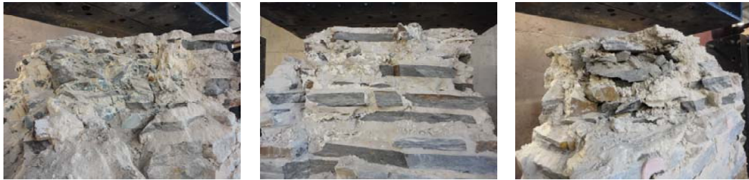
Figure 7: Appearance of the interior of the wall after dismantling: (a) P1; (b) P6; (c) P4
