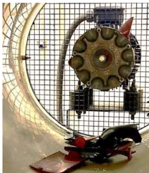
Figure 37-a. Accidental breakage of fan propeller.
