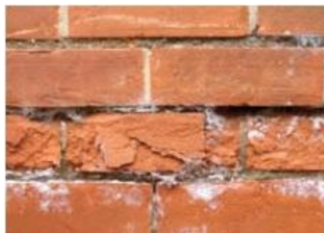
Figure 7-Salt attack in bricks causing damage.
