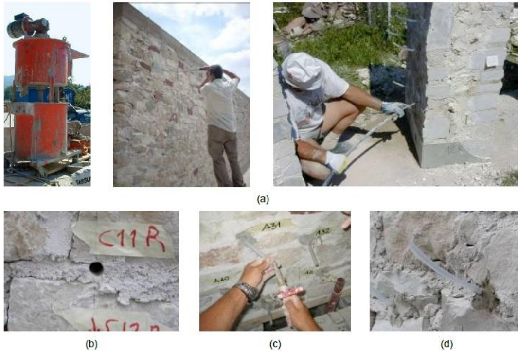
Figure 2-Grout injection procedure. (a) General overview of the process. (b) Drilling holes in mortar joints. (c) Fixing plastic pipes. (d) Injecting grout
