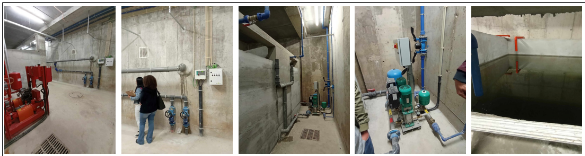
Figure 1 - Study visit to the rainwater harvesting system.
