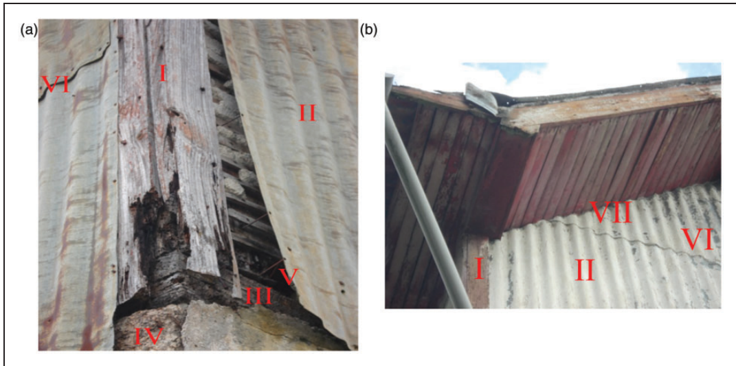
Figure 4. (a) Junction of walls and (b) roof abutment building details of the metal corrugated sheet coating. I: junction of tabique walls; II: metal corrugated sheets; III: timber frame; IV: granite masonry wall; V: nail; VI: connection of sheets; VII: roof abutment.
