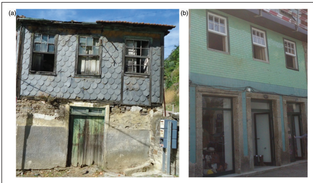
Figure 3. (a) Slate boards and (b) ceramic tiles as exterior types of finishing of Portuguese tabique dwellings.
