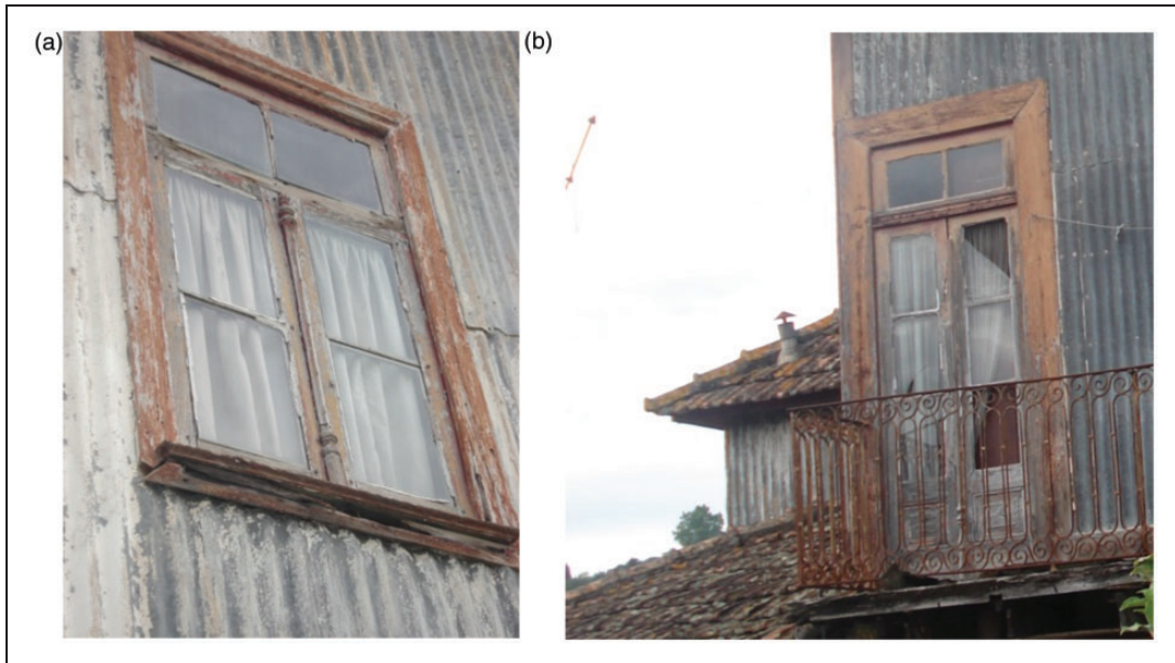
Figure 5. (a) Window and (b) door abutment building details of metal corrugated sheet coating.
