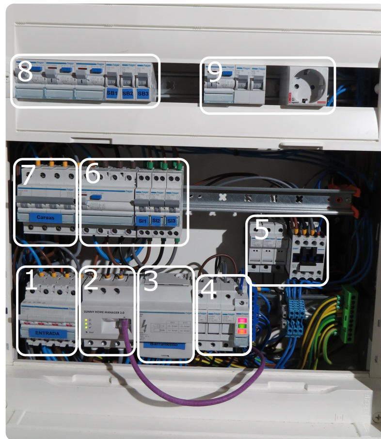
Figure 4.17: Electrical panel with devices of the microgrid.
