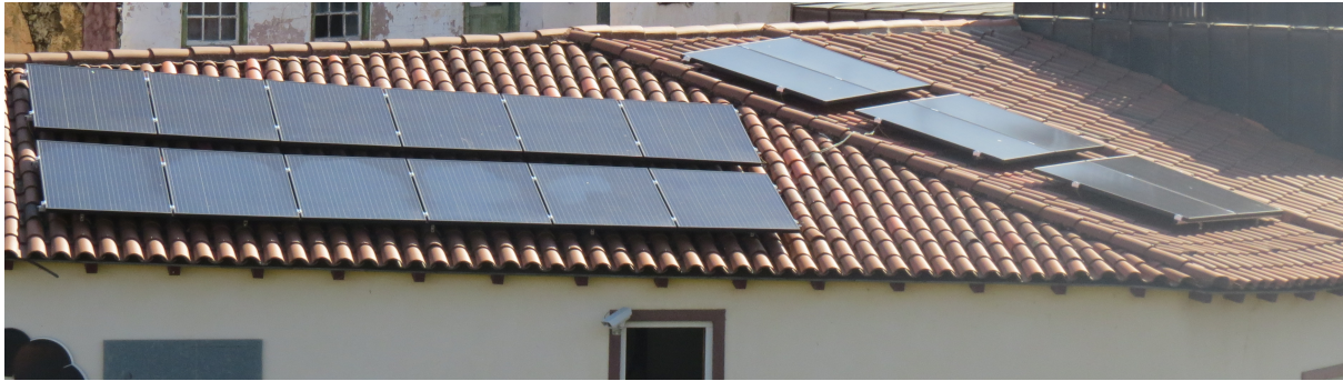
Figure 4.12: Photovoltaic modules installed in the Silk House.
