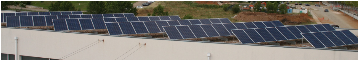
Figure 2.2: Photovoltaic modules installed at the ESE rooftop.
