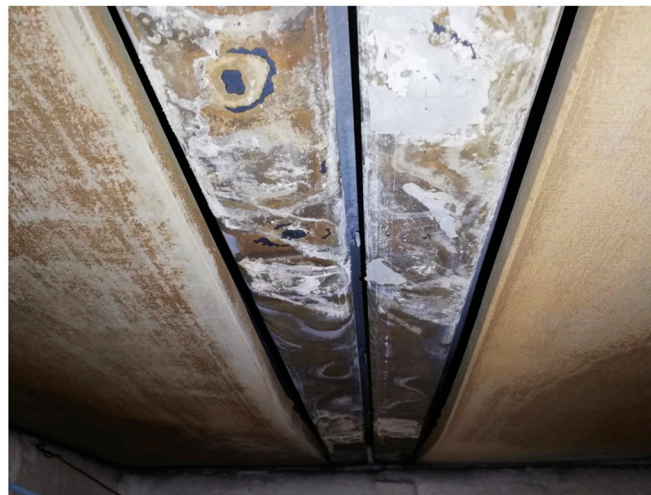
Figure 6. Specimen 2, obtained from Fourie [21], after the test was completed.
