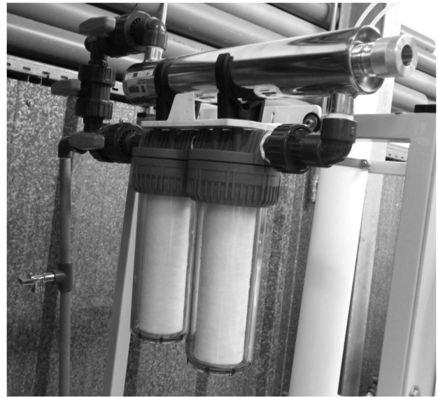
Fig. 5. UV disinfection system.
