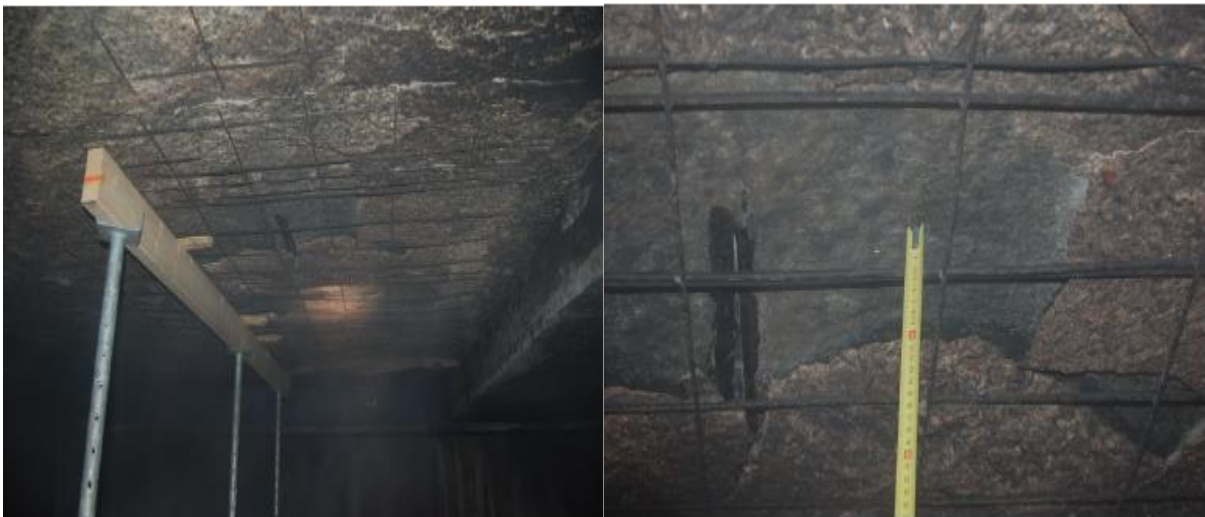
Figure 9: Structural damage after the cars fire in car park at Ruitersstraat Hilversum. [13]
