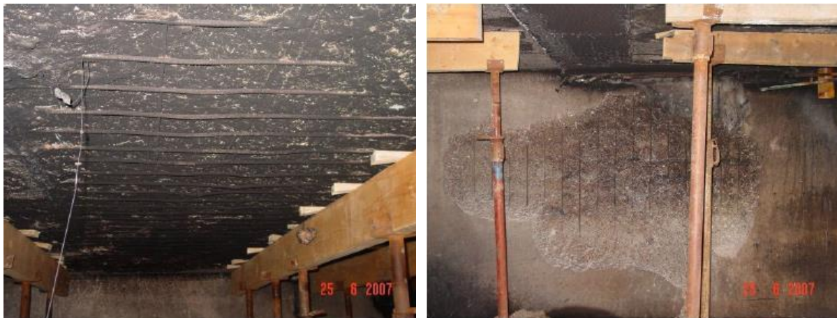
Figure 2: The Geleen car park after the fire. [15]
