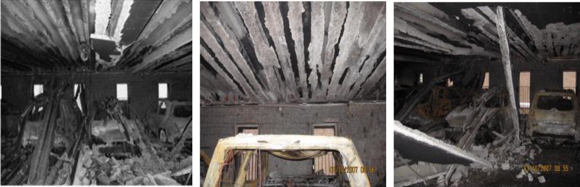
Figure 7 : Collapsed bottom halves of hollow core slabs of the building Harbour Edge. [17]
