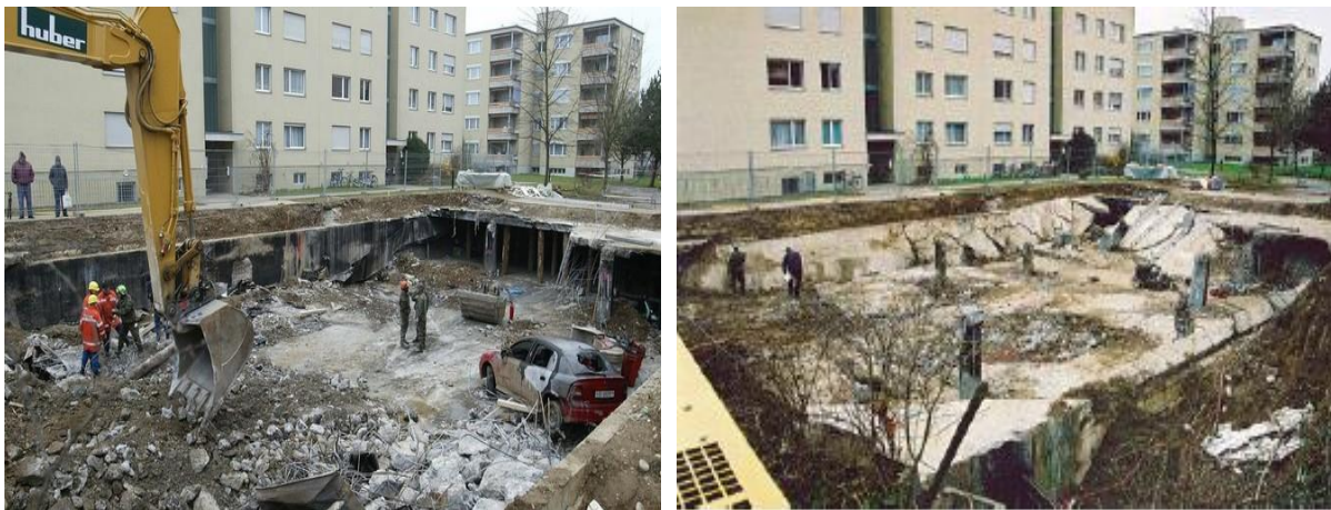
Figure 3: Gretzenbach underground car parking 2004. [17]
