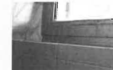
Presence of molds in a window located in the warehouse
