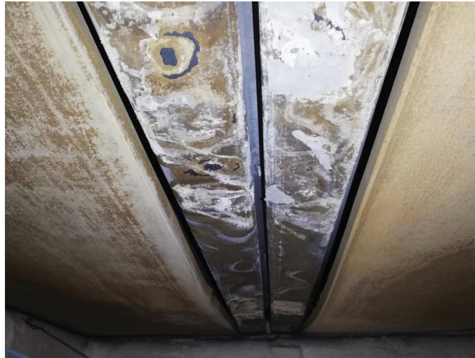
Figure 6.1. Specimen 2, by Fourie [15], after the test was completed.
