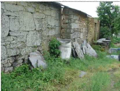
Figure 6. Posterior façade without connection and continuity.
