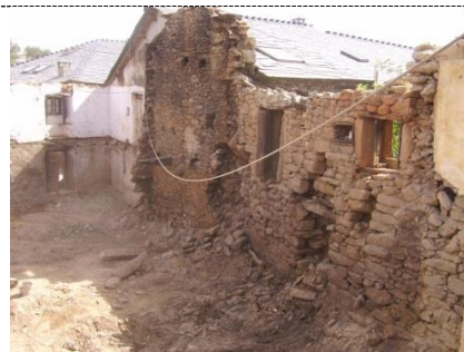
Figure 7. Adjoining building façades with little stone pieces. Electrical cables networks crossing the building
