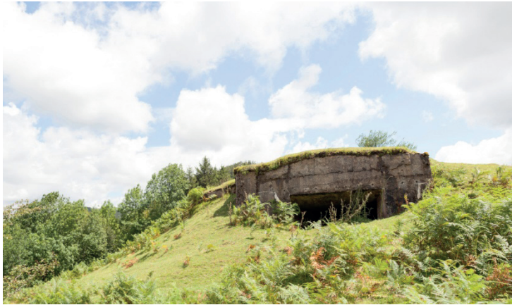
Figure 2: Military bunker of the P Line in the Pyrenees. Otxondo (Baztán – Navarre). Picture by Carlos Orduna Portús
