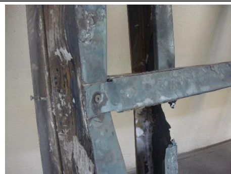
Distortional buckling in stud C (mid-height)
