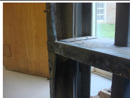
Distortional buckling in stud C (mid-height)
