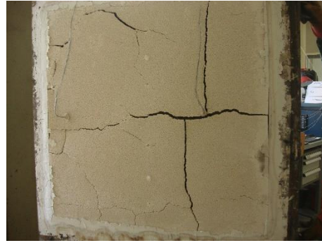
Cracks on the exposed surface
