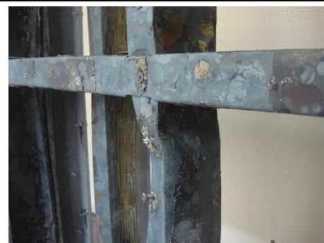
Web buckling in stud B (mid-height)
