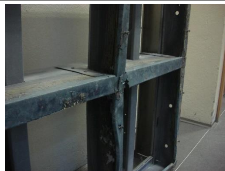
Web and distortional buckling in stud B (upper part)
