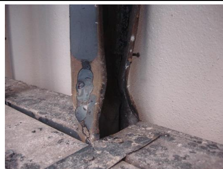
Distortional buckling in stud B (upper portion)
