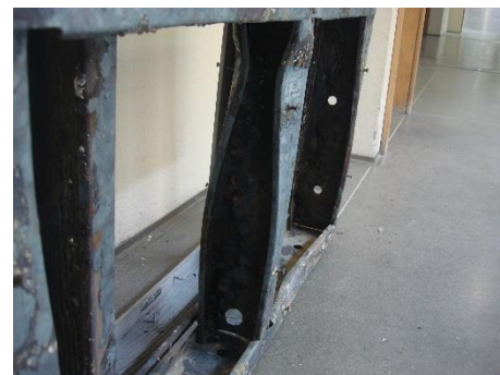
Distortional buckling in stud B (lower part)
