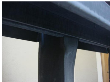
Web and distortional buckling in stud B (top)
