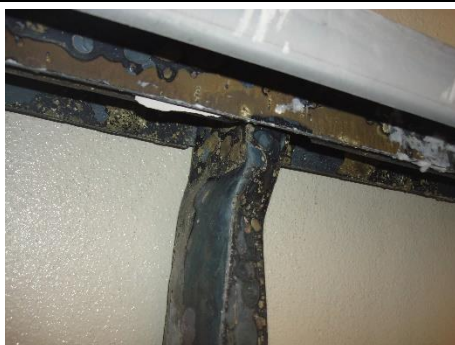
Web buckling in stud B (upper part)
