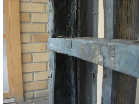
Distortional buckling in stud C (mid-height)
