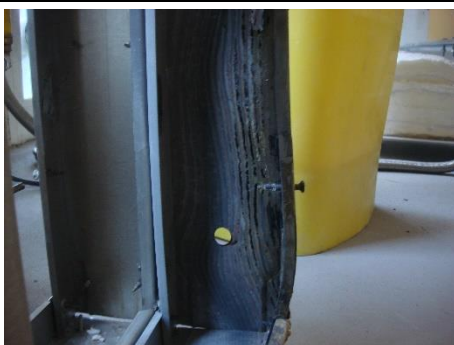
Distortional buckling in stud A (lower part)
