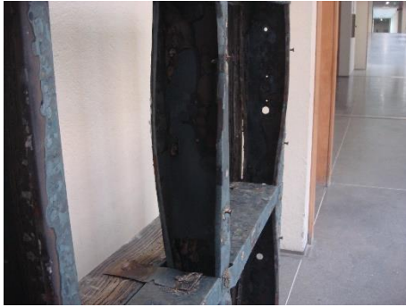
Distortional buckling in stud A (mid-height) and stud B (upper part)
