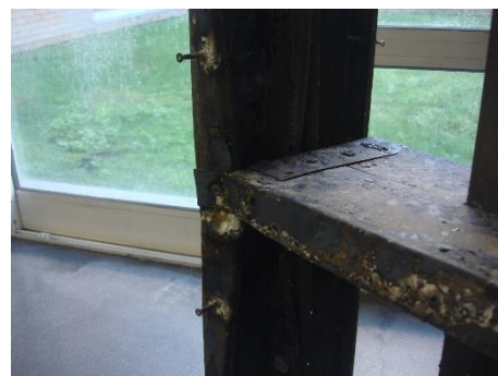
Distortional buckling in stud C (mid-height)
