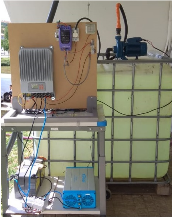
Figure 4.9: Experimental platform for low power applications based on the integration of a charge controller, a battery, a battery inverter and a SFC.
