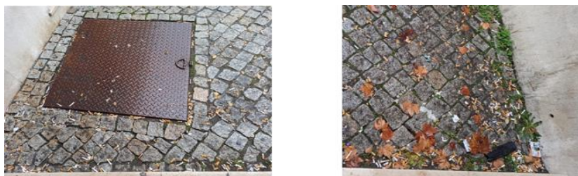
Figure 1 The external floor of the Higher Education School before the intervention (photograph taken by the authors)
