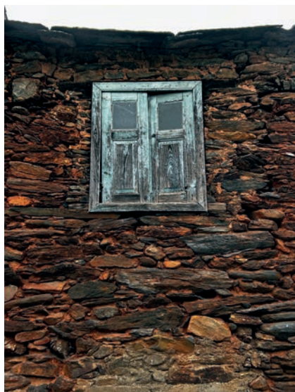
Figure 14. Timber in windows
