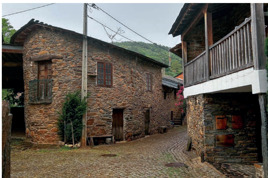
Figure 1. Influence of colour and texture of the chloritic or micaceous schist strongly in the aesthetic of façades
