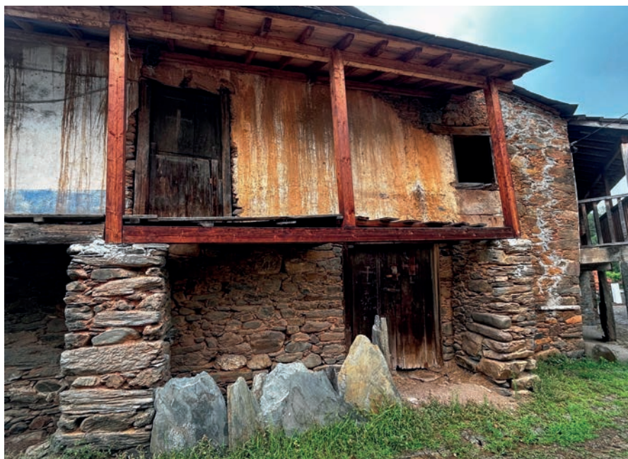
Figure 12. Balconies, porches, and window frames
