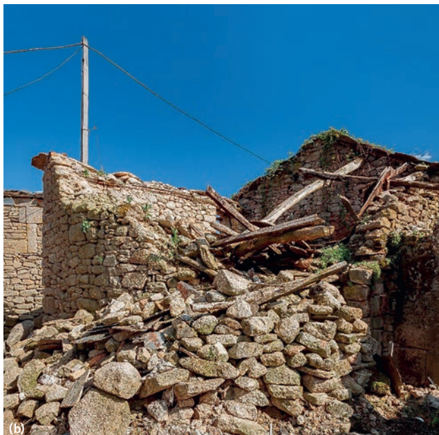
Figure 13. Building collapse record: (a) initial state (2023); (b) ruin state (2025)
