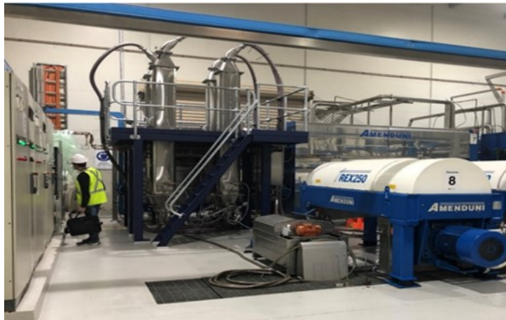
Figure 2.20: Megasonic reactor set for operation [4].
