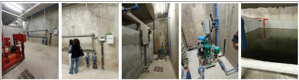
Figure 1 - Study visit to the rainwater harvesting system.
