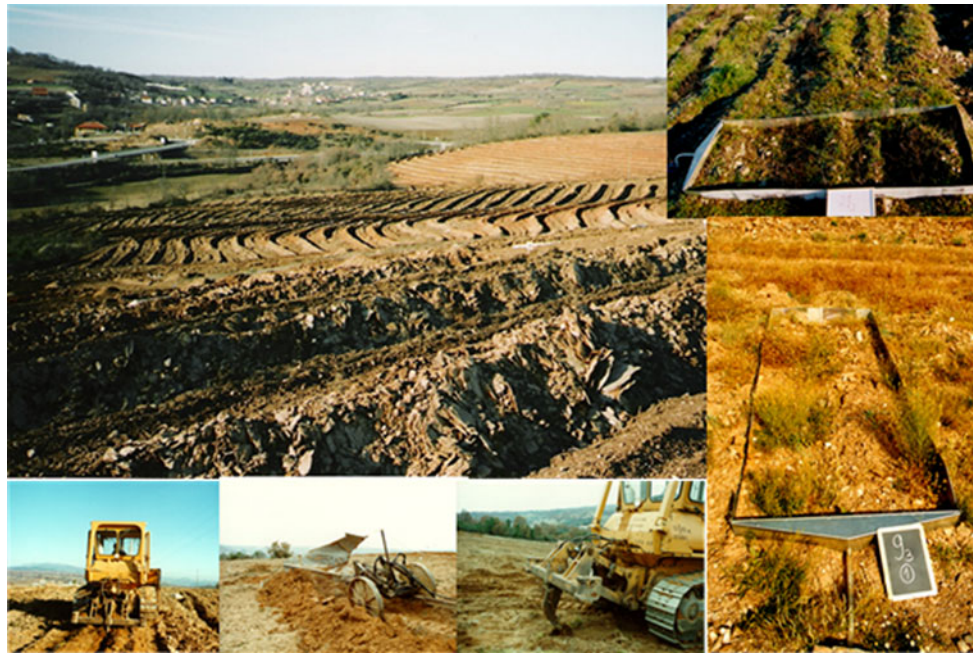
Photo 1 Experimental area: general view after site preparation (contour bunds freshly shaped, with evident soil disturbance and exposed rock fragments) ( centre ); machinery operating and some
