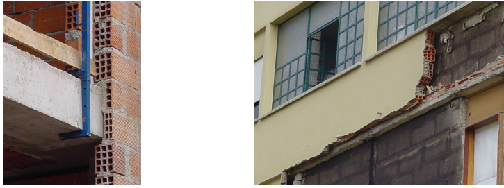
Fig 2: Deficient brick covering on the edge of a beam creating insufficient width support of the exterior leaf and the collapse of an outer leaf.
