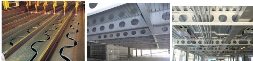
Figure 2 - The cutting process of cellular beams. The use of cellular Beams in buildings, [2].
