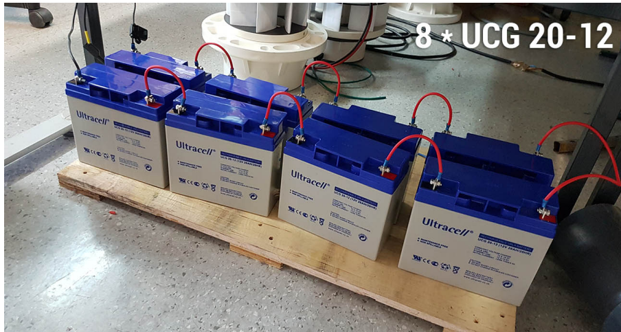
Figure 4.14: Ultracell UCG20-12 batteries.
