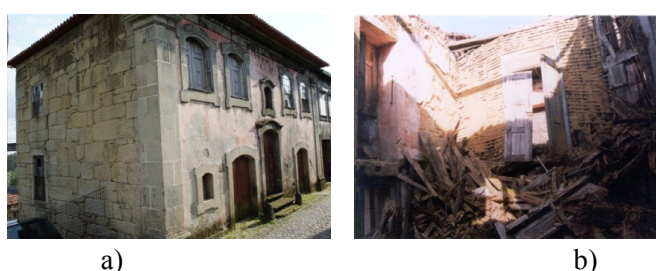
Figure 3: a) Building exterior walls; b) Interior building degradation and ruins
