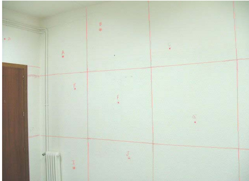
Figure 5.3 – In situ , “Magisterio” receiving room measurement surface separating element, divided on twelve sub-areas
