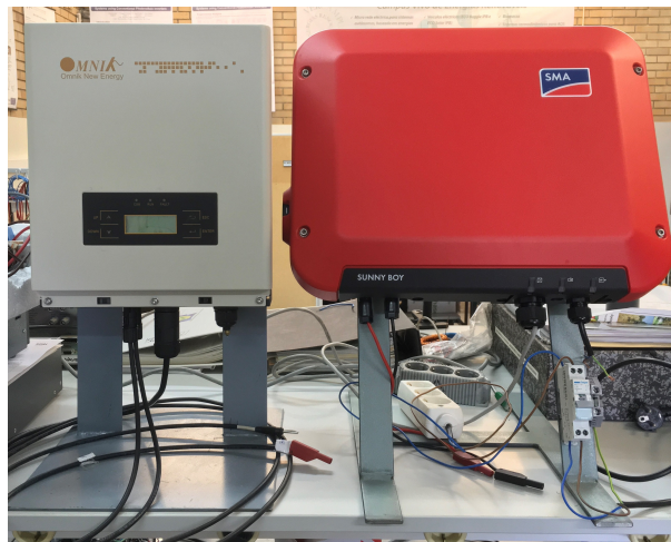
Figure 2.6: PV inverters: Omniksol-2k-TL2 (on the left) and SB 1.5-1VL-40 (on the right).
