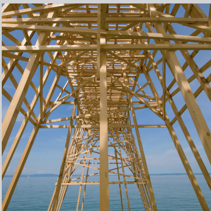
... Timber Bridge Construction in Arbon, Bodensee in Steinach, Canton of St. Gallen, Switzerland. (Copyright Norlando Pobre, www.flickr.com : CC-BY)
