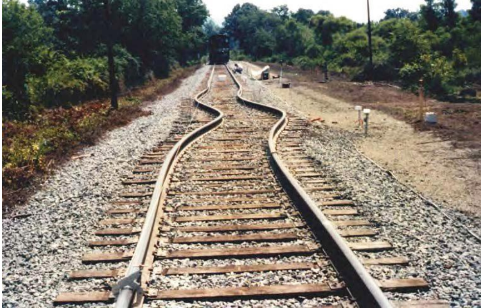
Figure 3.14 - Deformed buckling mode (III) to tangent railway track [18].
